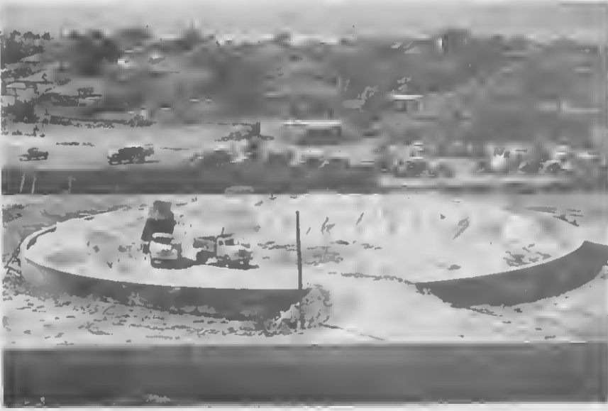
2 SAND IS needed to form a solid packed base. Depending on the elevation of the site up to 10 feet of sand was poured. TIN MESTER di santo pa forma un hase bon pilá. Dependiendo di elevacion di e sitio entre dos y 10 pia di santo mester a worde bashá.
